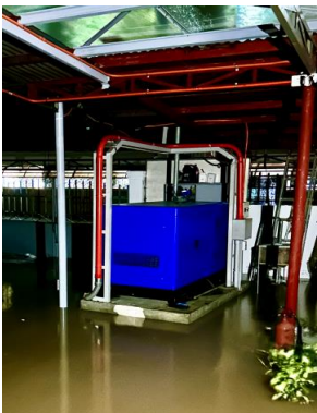
High flood waters nearly reach the campus generator.
