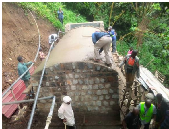
The new water tank to supply water for the hospital during dry season to now be linked with the UV filtration system.
