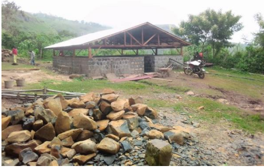
New roof now covering both the old and the new upper water filter houses. The UV treatment units are there and will be installed as well in the lower filter house. This should more than double the production of water at the end of the dry season.
